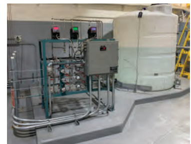
SCR with Non-Hazardous Urea
